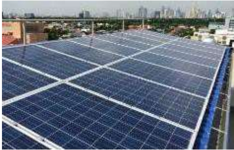
Taguig rooftop PV project
