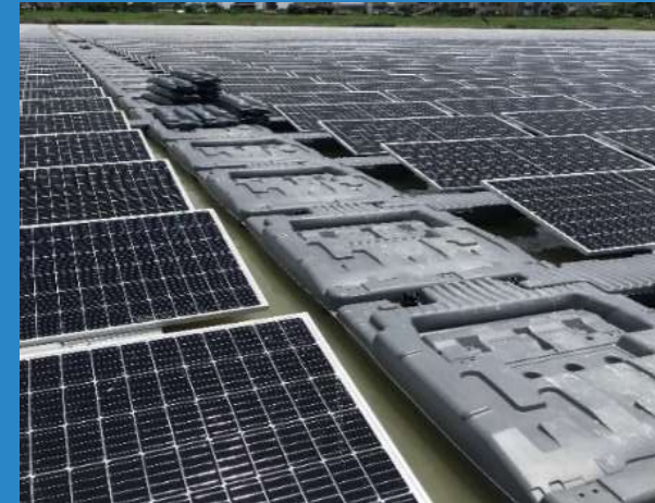
7 MWp Array, Taiwan; Source: MM
