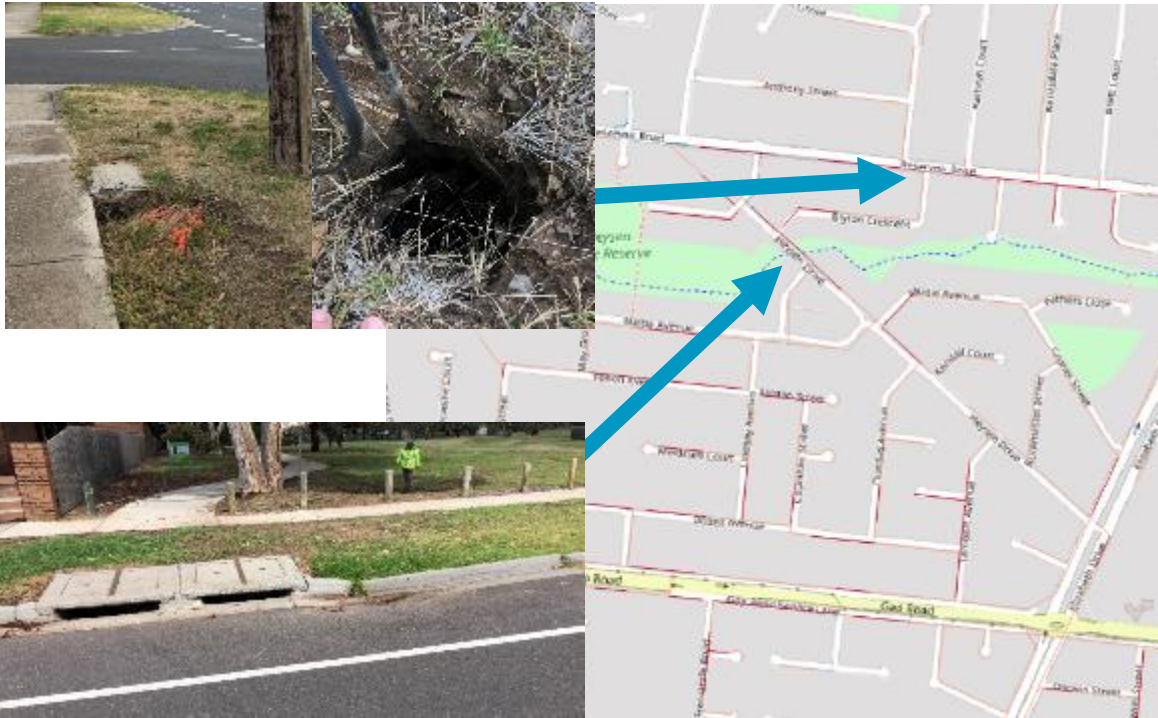
Subsidence around drainage covers - 65 Heysen Drive
