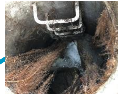
Root intrusion Cnr Elizabeth & Menzies Drive
