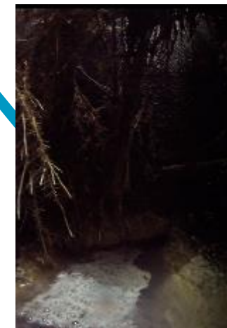
Elizabeth & Menzies Drive, partial blockage due to root intrusion
